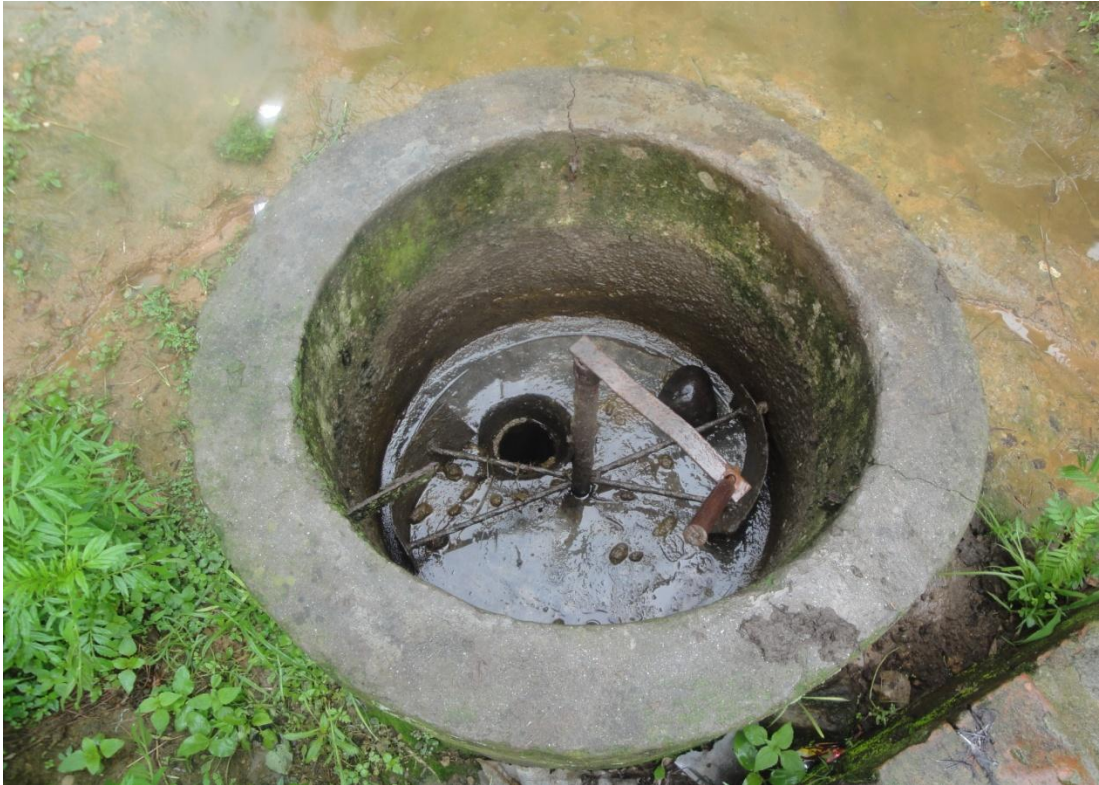
Figure 9. Intake of Feeding Material in Biogas Plant
